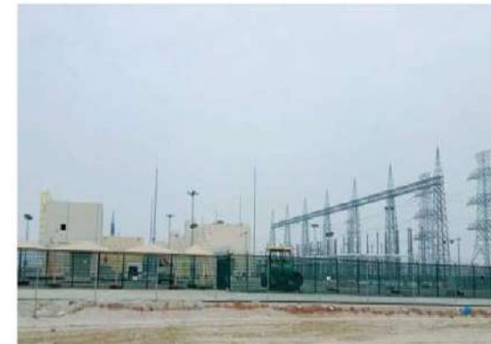
SEC 380kv Substation, Marjan, Tanajib
